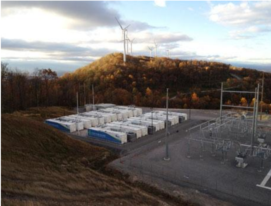
Photo: AES Energy Storage
